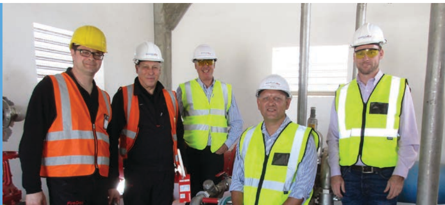
Commissioning Cape Town harbour sea water FD20000/1/3 foam proportioner with Ingo Wosch and Heinrich David, the founder of FireDos (on the left), Mike Feldon, JB Potgieter and Greg Buchanan from DoseTech
